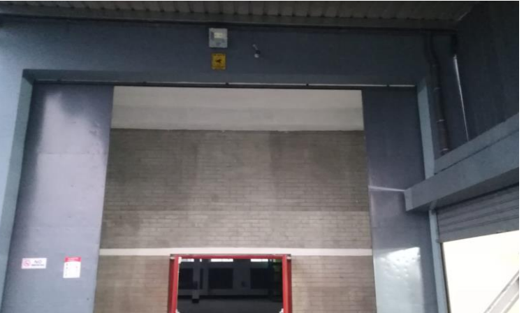
Multi Layer Secured Entrance
