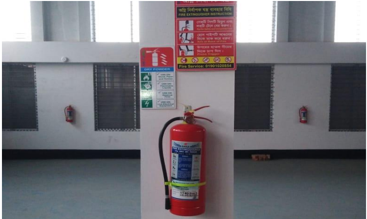
Fire Extinguisher (Manual)
