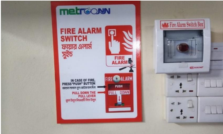
Fire Alarm Switch
