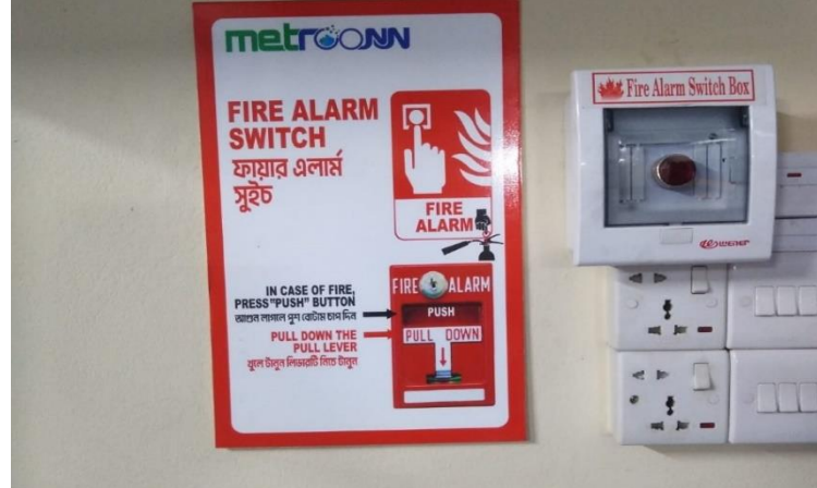
Fire Alarm Switch
