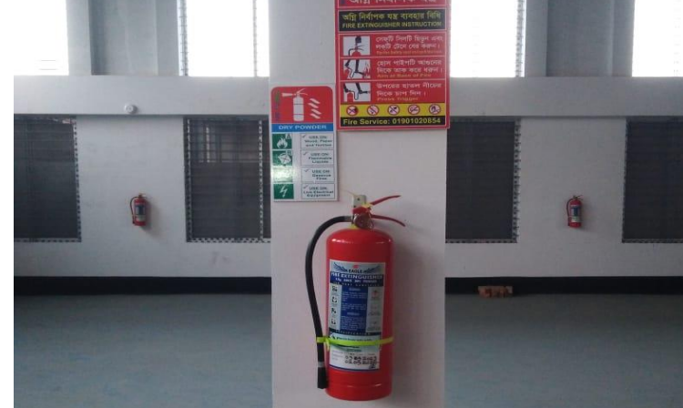
Fire Extinguisher (Manual)
